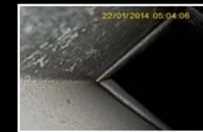
Internal duct work using 28mm detachable camera head (VSC28)
